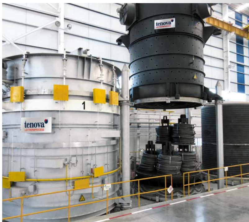
▲ HPH® Bell-type Annealing Plant for CHQ wire
